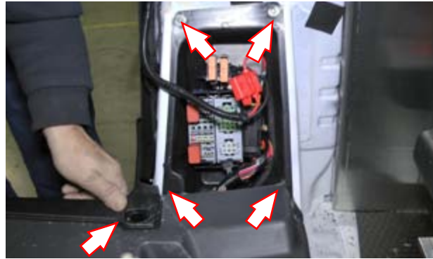
Distribution panel and stepwell screws
