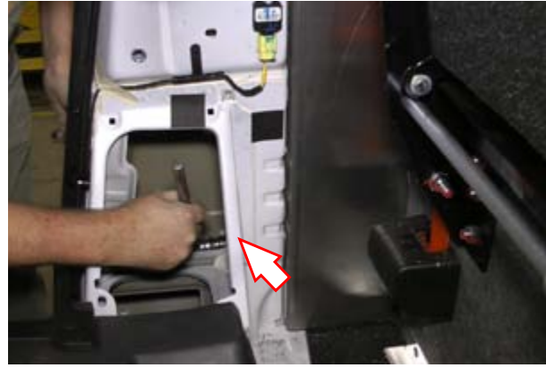
Nut and washer inside distribution panel
